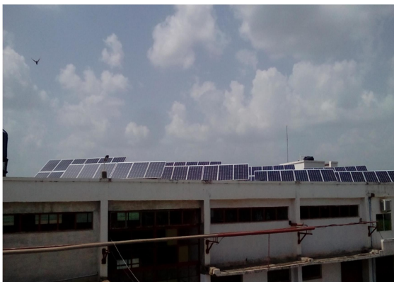
Malabar Dairy, 30 KWp Solar (Off Grid) Rooftop Power
