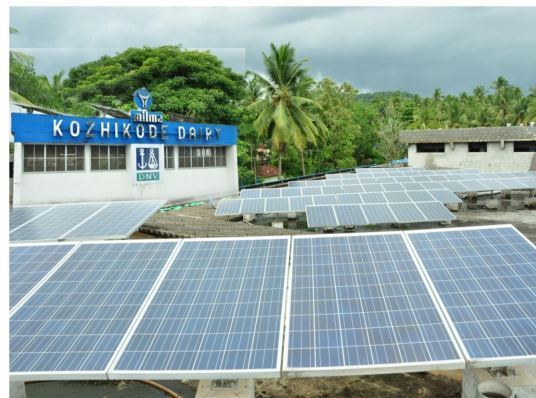
Parvati Dairy, 100 KWp Solar Grid connected Rooftop Power
